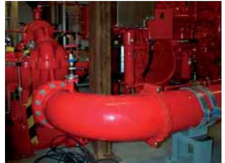
Alvenius® Thermoplastic Coated pipes are used in the fire protecting system at Ringhals nuclear power plant, Sweden.
