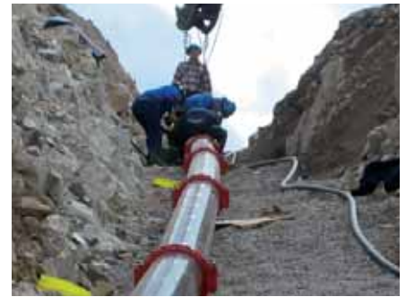
Installation of pipes for water supply to the snow guns. Idrefjäll Sweden.
